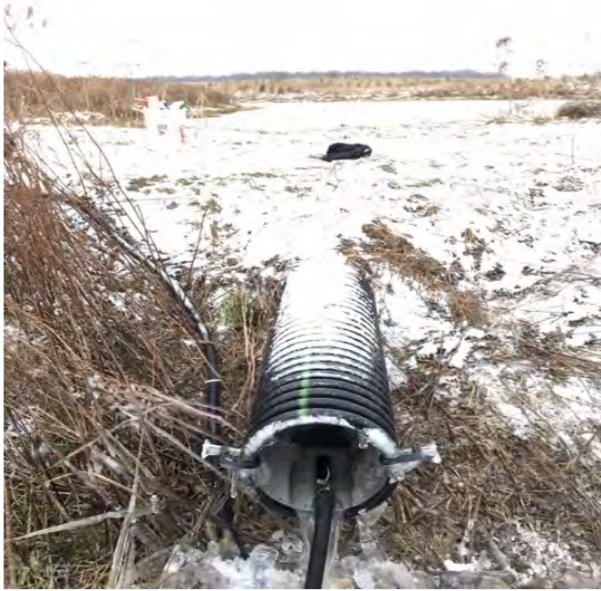
Figure A 18. Deployed area velocity flow probe collecting flow data every 15 minutes at the outflow of site KE.
